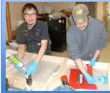
Demetri Gust (left) working on air sealing penetrations while Jerry Gust (right) air seals a break in the vapor barrier during a Weatherization Tech 1 class held in New Stuyahok, October 2012.
